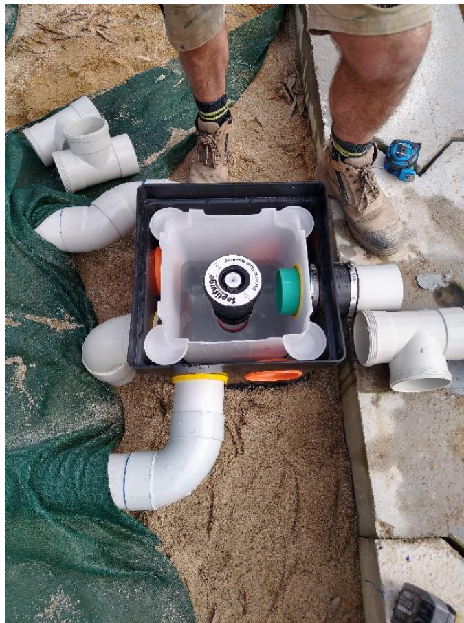
Figure 2. Photograph of SeptiSurge® dosing siphon distribution box supplying influent wastewater to the Eljen GSF advanced secondary system.
