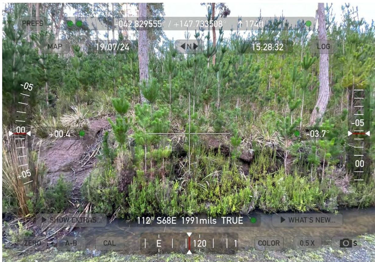
Photo 20 - Erosion next to table drain
