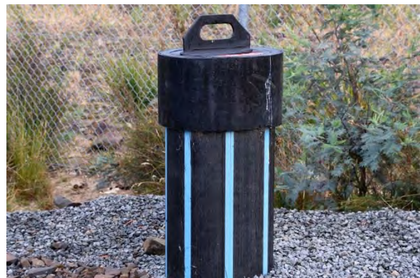
SS8: C-Cell LBP-Seepage Pit
