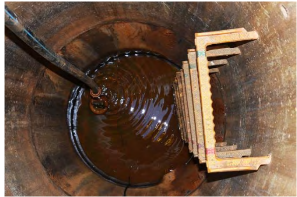
SS4: PLP Underliner Drainage Pit
