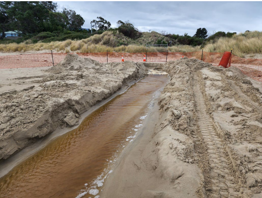
Figure 7: Outfall in the Blue Lagoon Beach to ease water from Blue Lagoon
